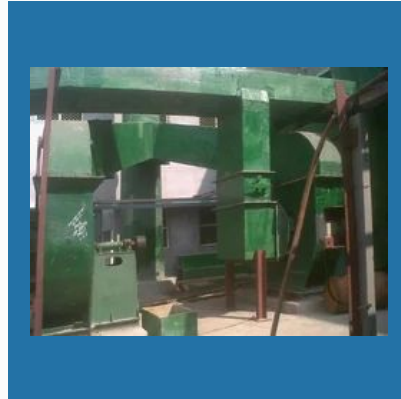
Chimney Ducting for Fumes Exhaust
