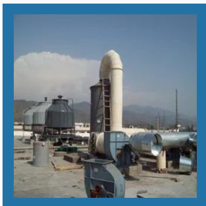
Fume Extraction Duct Units
