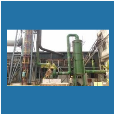
Chimney Ductings for Fumes Exhaust
