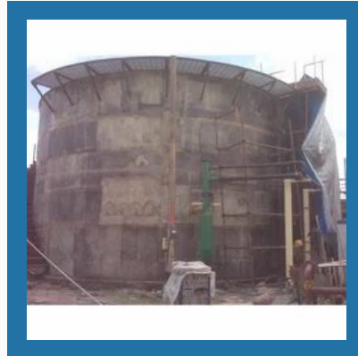
Effluent Treatment Plant Tanks
