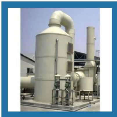
Acid Fumes Exhaust Systems
