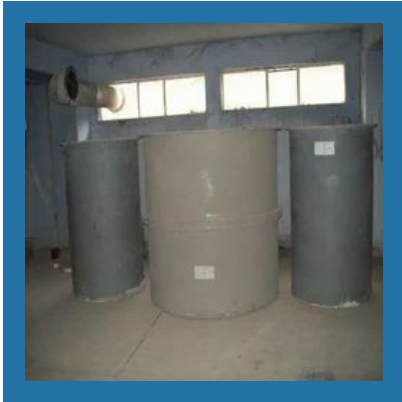
Industrial Acid Dosing Tanks
